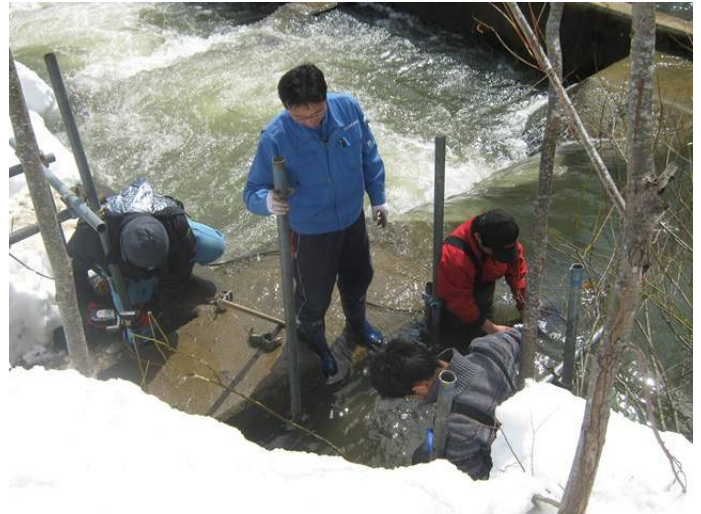
With the help of members of Sarufutsu Itou no kai , we built a frame to support the sonar system. Photo credit: Pete Rand
